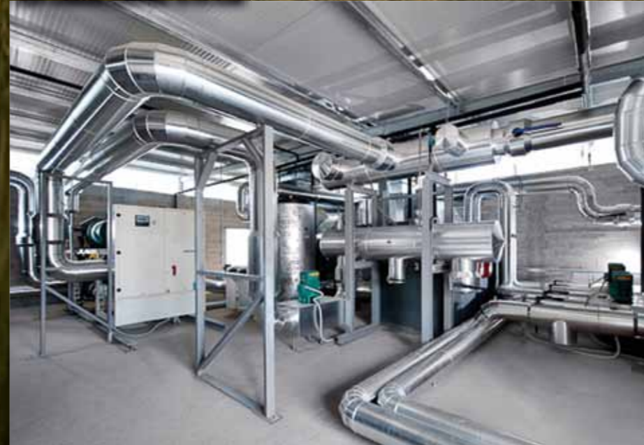
AIR CONDITIONING SYSTEM
